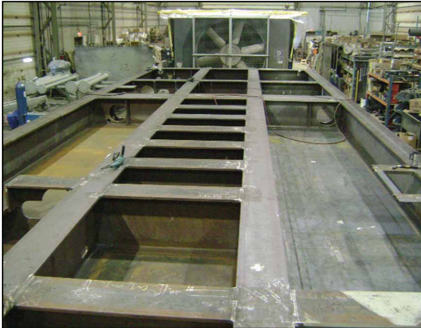
The 740 hp (550 kW) skid, with a total length of 56.5 ft. (17.2 m), required extra heavy-duty 24 in. (610 mm) steel I-beams to address package deflection. All critical skid welds were ultrasonically tested to ensure their integrity.
